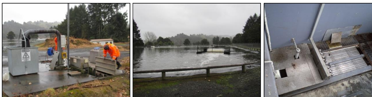
Figure 13 Treatment plant examples
