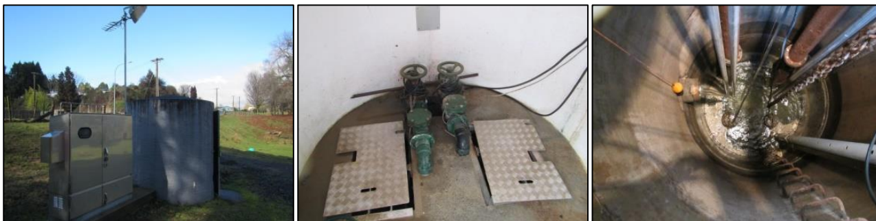
Figure 12 Pump station examples
