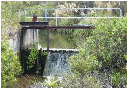
Ohakune Raw Water Intake
