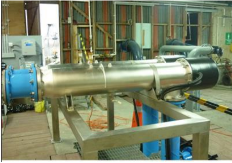
Matapuna WTP UV units
