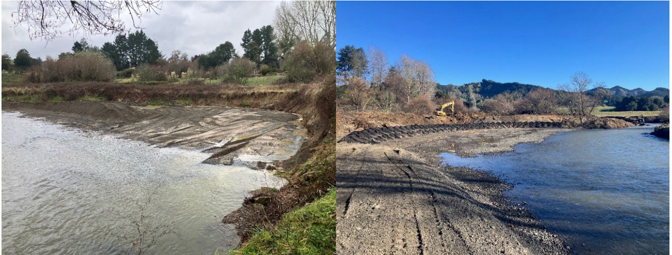
Eroded land with landfill in back ground being prepared Te Horangapia being protected by rock bags for protection
